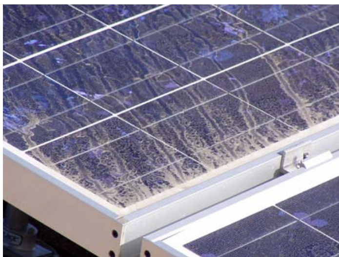
Fig. 2 Dust fall on solar panels.
