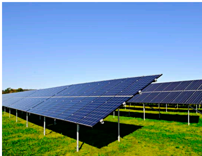
Fig. 3: A clean and functioning solar installation
